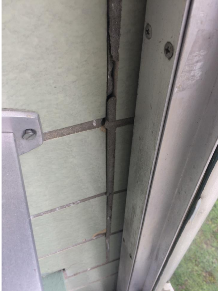
Interior wall cracks
