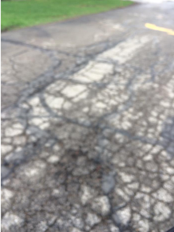
Asphalt in poor condition
