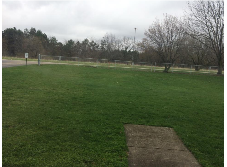
Fencing in poor condition
